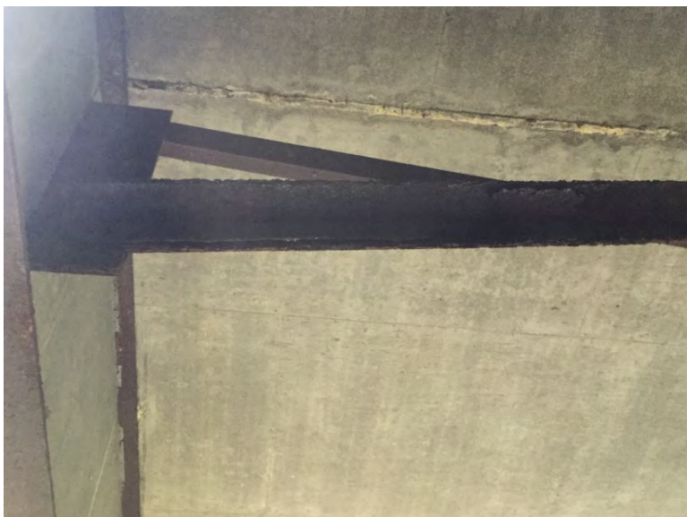
Corrosion noted on center diaphragm
