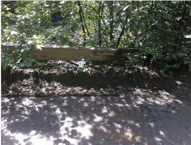
Sediment on deck and damaged guardrail
