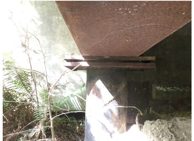
Slight bulging of bearing pads
