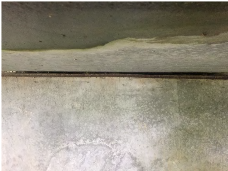
Slight top flange deformation noted downstream left bank
