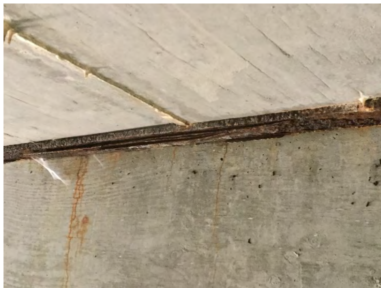
Corrosion of girders noted at deck panel joints
